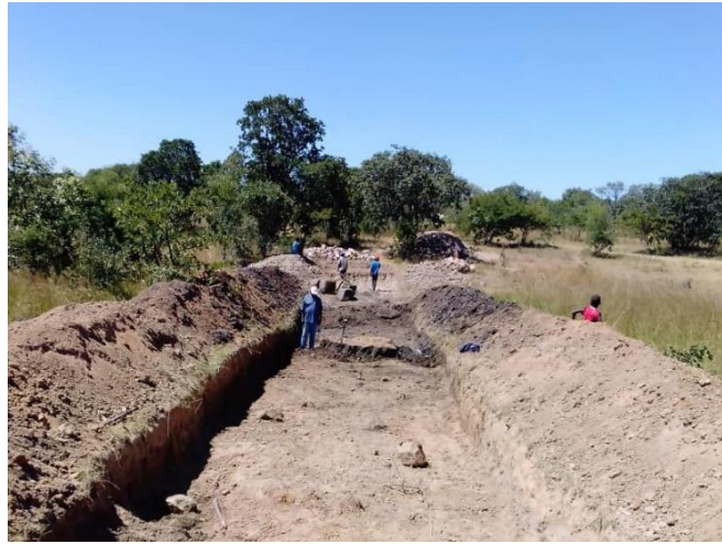
The excavation for the foundation and the construction of the dam was a joint effort of more than 65 people.
